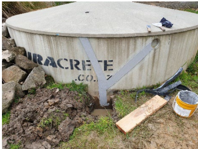
Repaired damage caused during backfilling
