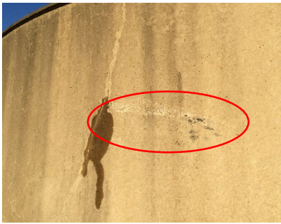
Damage caused during backfilling (impact point)
