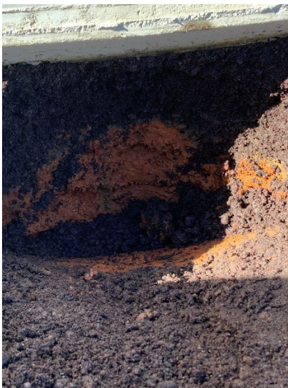
Inadequate site preparation showing fines sitting directly on clay. A 100mm compacted layer of GAP40 fill should be between the clay and the fines as per below:
