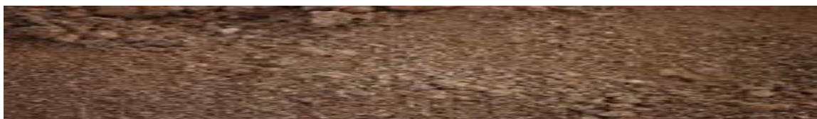
4.2m square excavated foundation. Levelled in all directions to a tolerance of 40mm. NZBC Clause B1.
