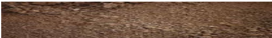
2.8m x 2m excavated foundation. Levelled in all directions to a tolerance of 40mm. NZBC Clause B1.
