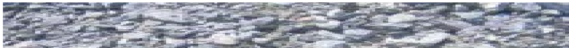
100mm layer of bedding material GAP20/7 (General All Purpose 7-20mm) to a tolerance of 15mm.
